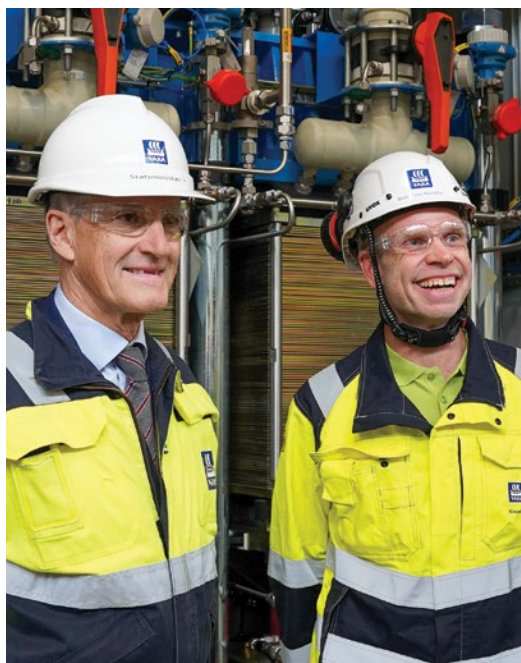
Norwegian prime minister Jonas Gahr Støre and Yara CEO Svein Tore Holsether at the opening of Yara's electrolysis hydrogen plant in Porsgrunn, Norway
